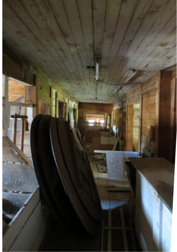
Photo 61: Later additions to the barn have little historic material for salvage. Not keyed.
