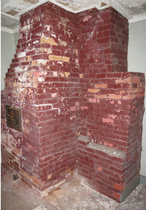
Photo 36: View of exposed chimney and early 19th century oven door in kitchen.
