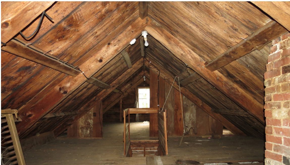
Photo 18: Old growth timber structural frame of house, rough-sawn wide sheathing boards, and historic brick in chimneys. Not keyed.
