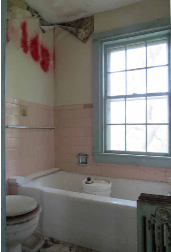
Photo 50: View in rear bathroom.
