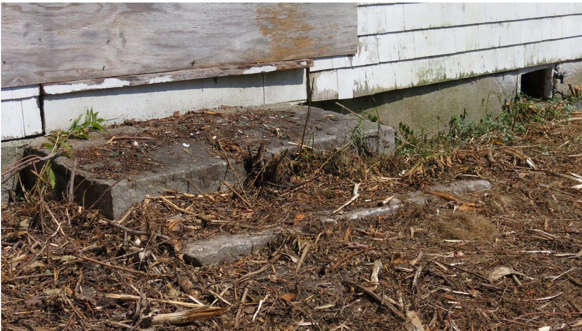
Photo 5: Granite steps at front and side doors, and granite cap stones on foundation.
